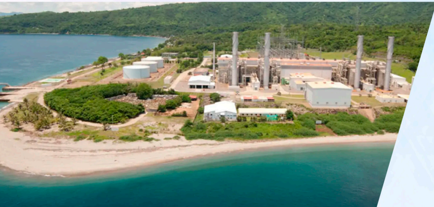
SAN MIGUEL CORPORATION Batangas Plant Products used: Confix L5, Cement Remover, Concrete Patch H, Confix LV, Confix IJ
