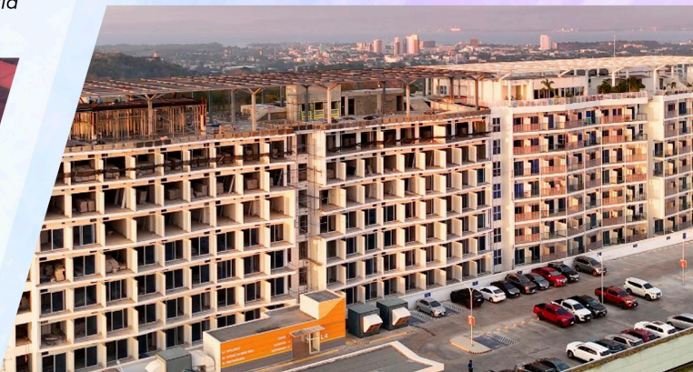
Citi Primavera, Cagayan de Oro City, Misamis Oriental Products used: Confix IJ, Confix HV, Concrete Patch V, Solidcure, Confix Anchor, Smartbond C1 and Putty Master
